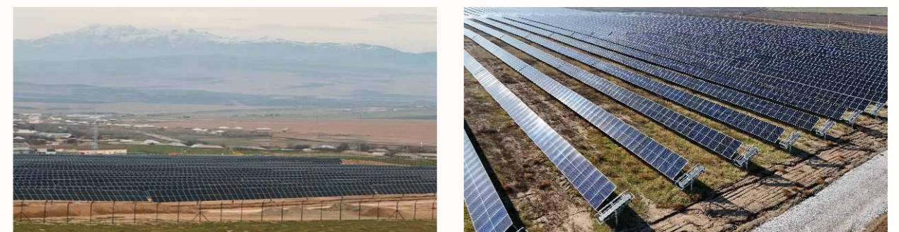
Uzbekistan 1 GW Utility-Scale Ground-Mounted Project
