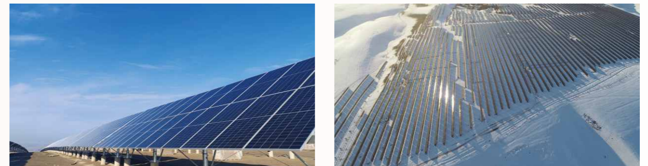
66 MW PV Power Generation Project of Yili Xintian Coal Chemical
